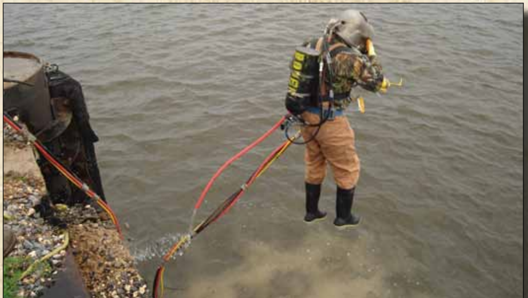
Colby Turner, Underwater Welder Global Industries Ltd., Sulphur, LA 2008 Welding Technology Graduate
